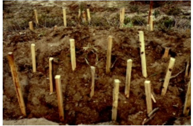
Figure 16-11b Each layer of branches is followed by a layer of compacted soil (Robbin B. Sotir & Associates photo)
