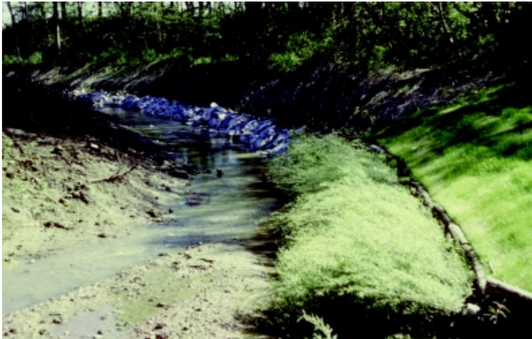
Figure 16-15c An established live cribwall system
