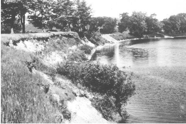
Figure 16-3a Eroding bank, Winooski River, Vermont, June 1938
