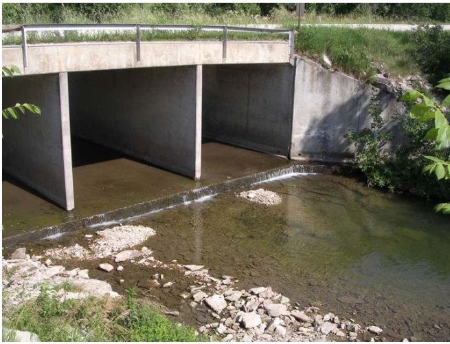
Figure 2. A box culvert with a waterfall at the outlet is a barrier to aquatic organisms swimming upstream.
