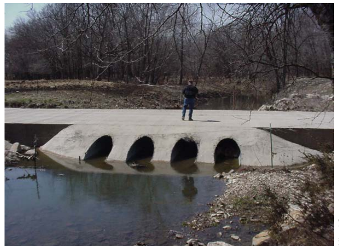
Figure 14. This low water crossing has larger vents that were set well below the channel elevation. This might be acceptable where there is little danger of channel incision for the life of the structure.
